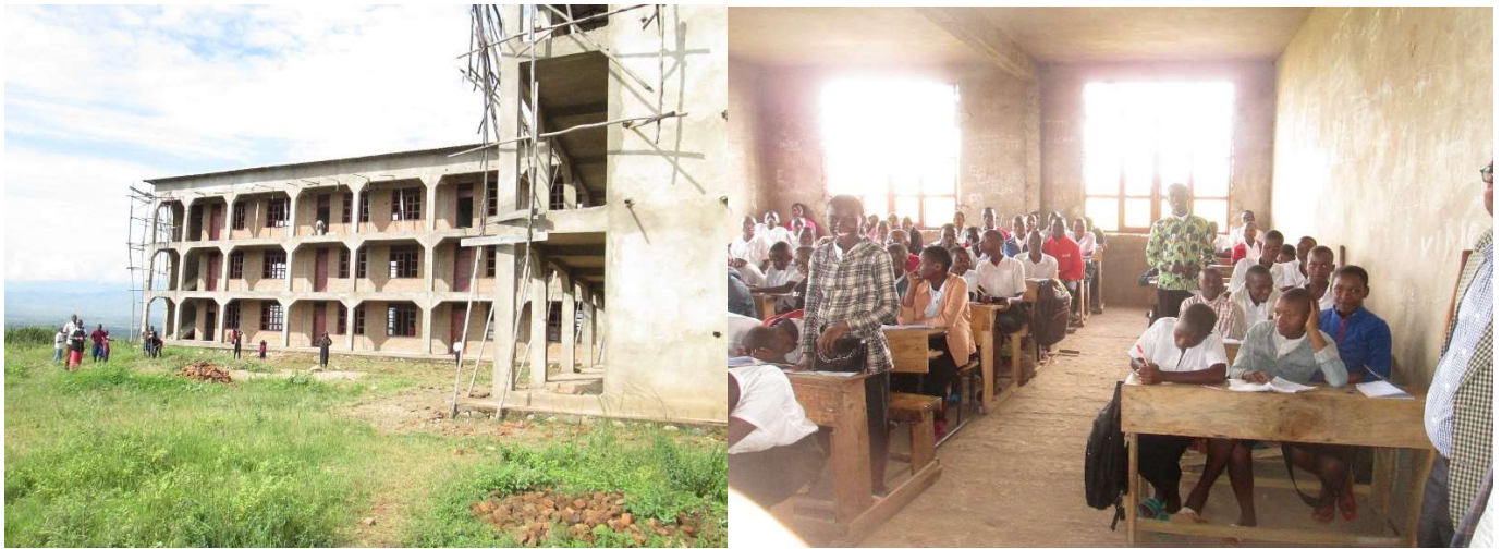
Cibitoke: the incomplete school building and a deaf class in an unfinished classroom
